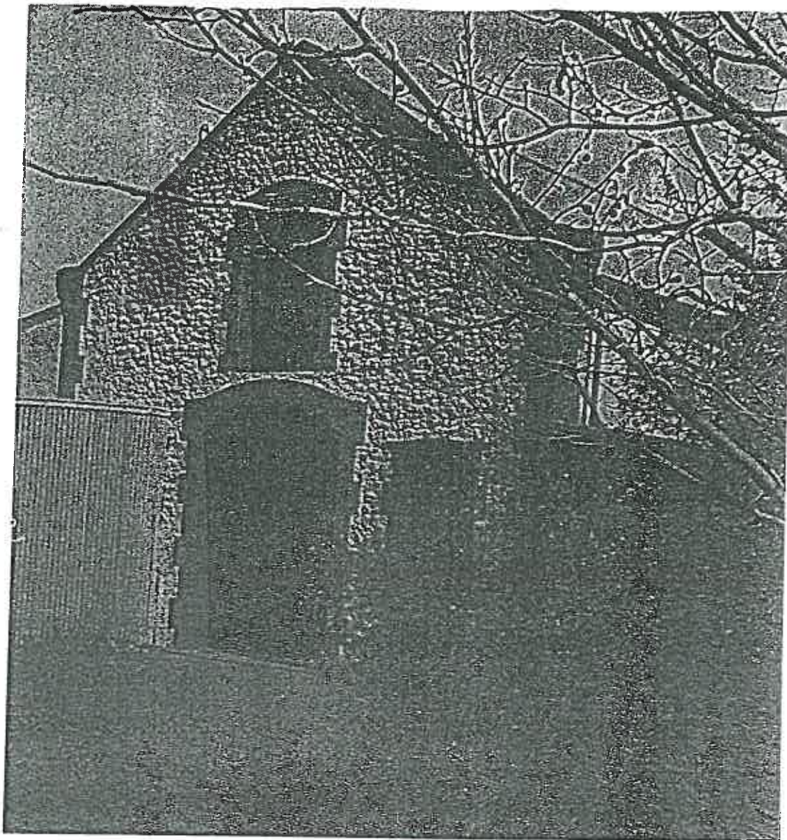
Fairford wine cellars built by William Henry Trimmer; later used as coach-house.
